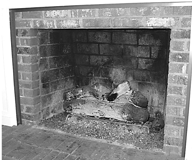
Masonry Woodburning Fireplace
