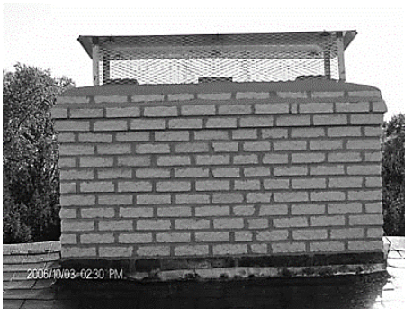
Metal Cap on Clay Liner Chimney Top
