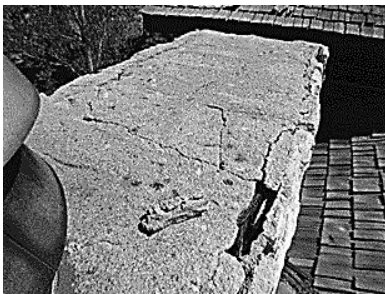
Damaged Chimney Cap
