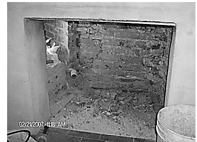
Badly Deteriorated Firebox
